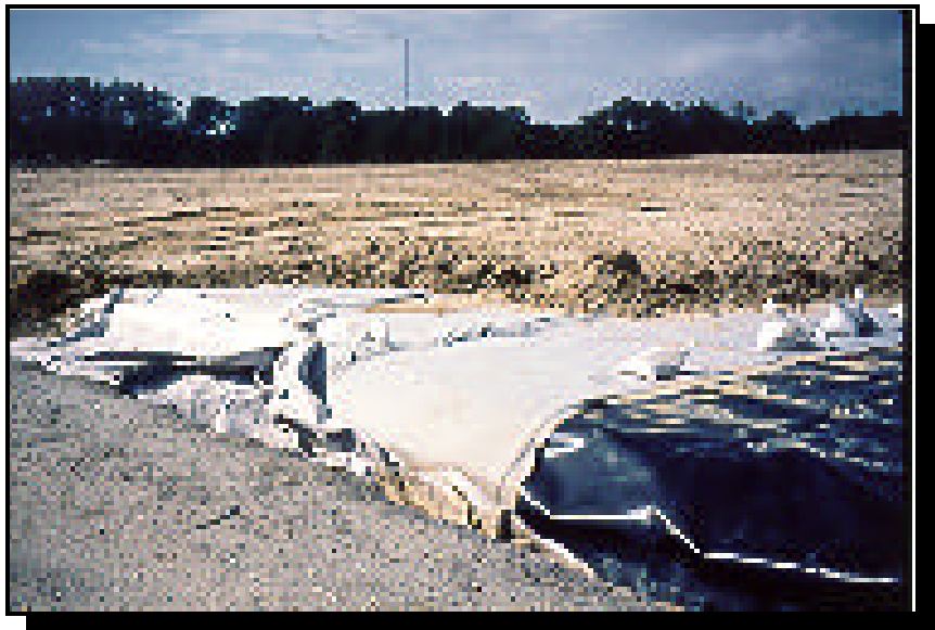
PHOTO #4 - Following thermal treatment the incinerator ash was placed in an onsite landfill, along with marginally contaminated soil and debris. An engineered cap was then constructed of high density polyethylene (HDPE), a geotextile material (Claymax) and native clay soil.
