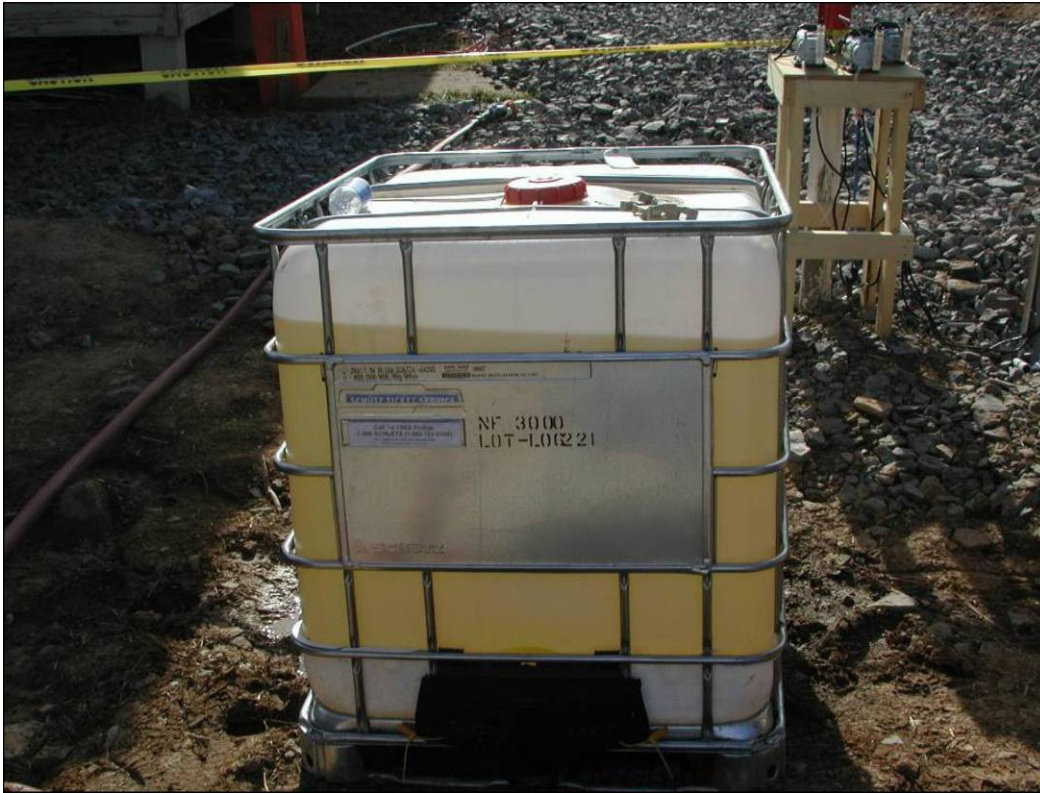
Figure 10. Wetting agent supply tank for the AACM demolition.
