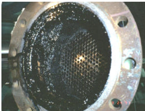
Figure 5. Tar condensed in water-cooled heat exchanger.
