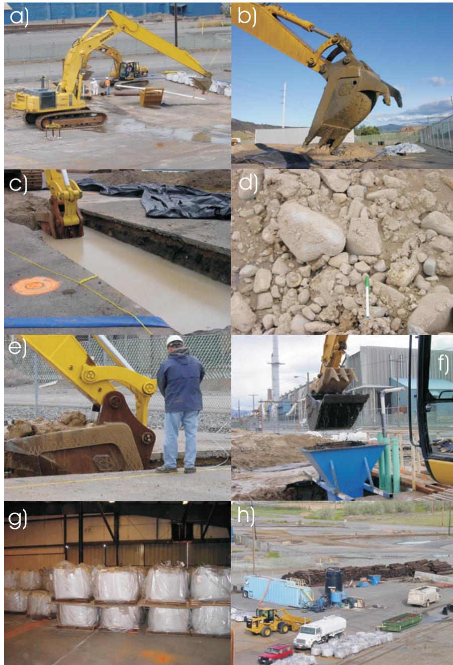
Figure 2. Installation photos: a) long-arm excavator, b) custom bucket, c) trench with biopolymer slurry, d) excavated materials, e) bucket with aquifer materials, f) tremie and trench backfill with granular iron, g) granular iron in super sacks, and h) construction site
