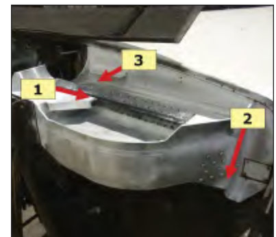
Talgo coach car tower support structure with locations of cracking identified.
