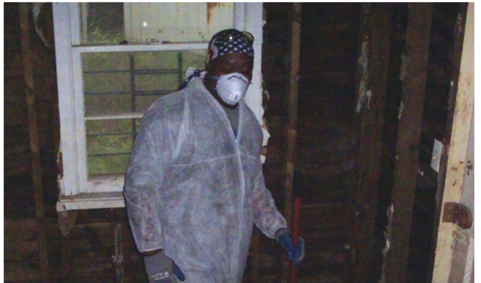
An AmeriCorps member with Trinity Christian Community in New Orleans guts out a house in the local neighborhood.
