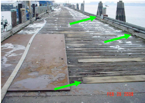
Highlight 12 shows the deck of Mallory Pier, the main training ship berthing pier. Metal plate covers large hole caused by rotten planks. Green arrows highlight (top to bottom) rusting 440v power terminal conduit; rotting power cable foundation; new planks installed to replace rotten planks over smaller holes.
