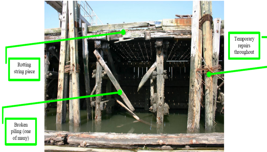
Highlight 14 shows deterioration of foundational structure comparison of Mallory Pier. Condition shown is typical of that found along the outer 700' section of the pier, which provides critical mooring facilities for the Academy's training vessels (224', 108', 65'), as well as mooring for the 4 vessels for USCG Station Kings Point.
