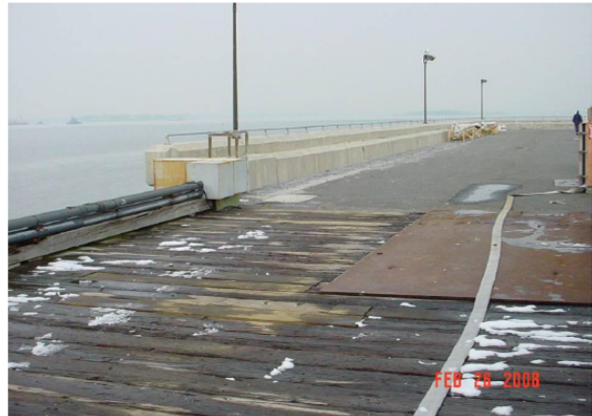
Highlight 13 shows comparison of old pier (foreground) to new pier (completed 2000). Concrete bulkhead provides additional protection to personnel and vessels from surf and spray. 400v power cables are also encased in concrete. Pier is basic and functional, with nominal lighting, handrails, and other required design elements.
