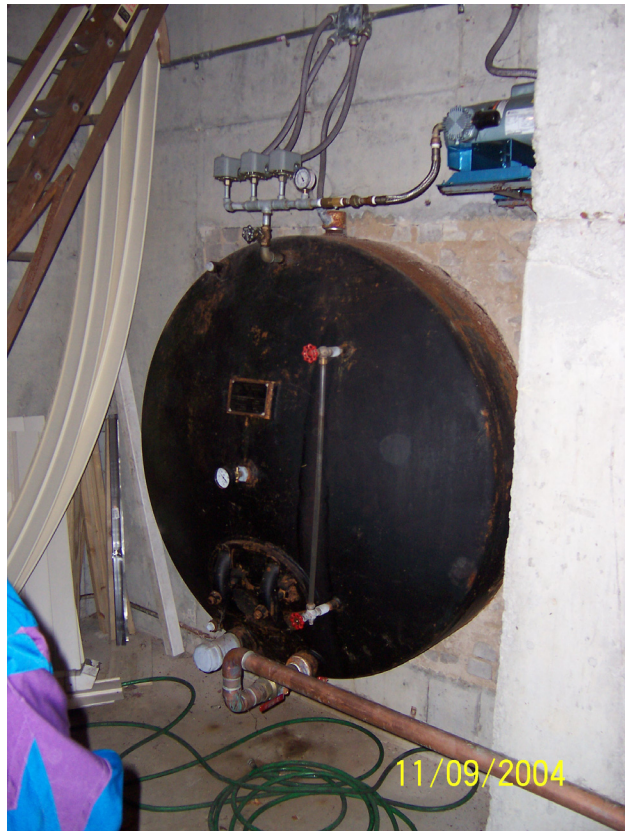
Figure 4-5. 2,000-gal Hydro-pneumatic Pressure Tank
