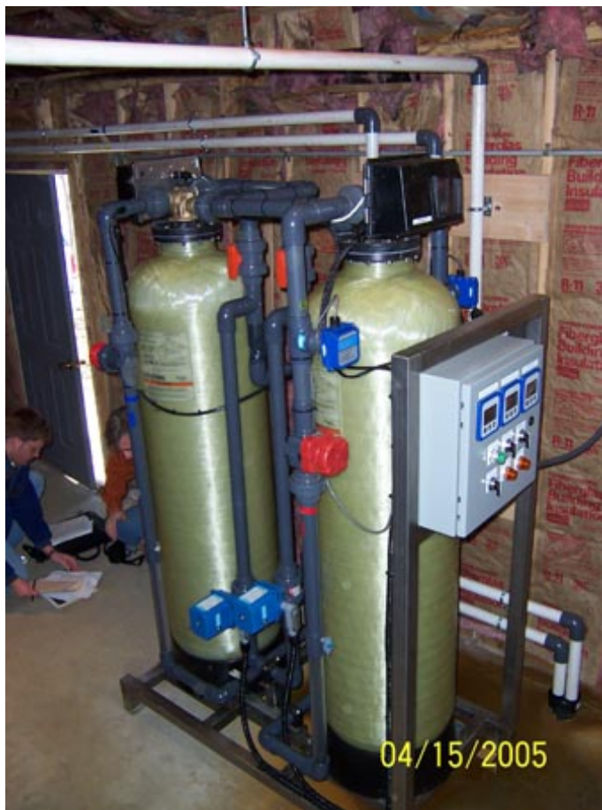
Figure 4-8. APU-GOFF-LL Treatment System
