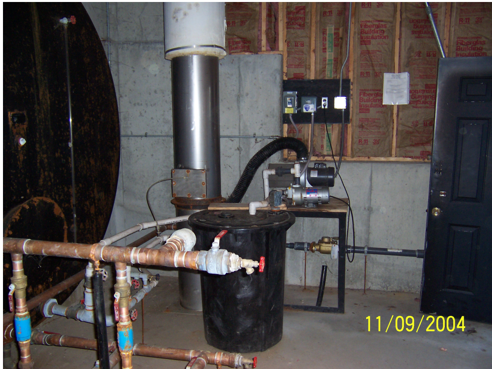
Figure 4-2. Aeration System for Radon Treatment
