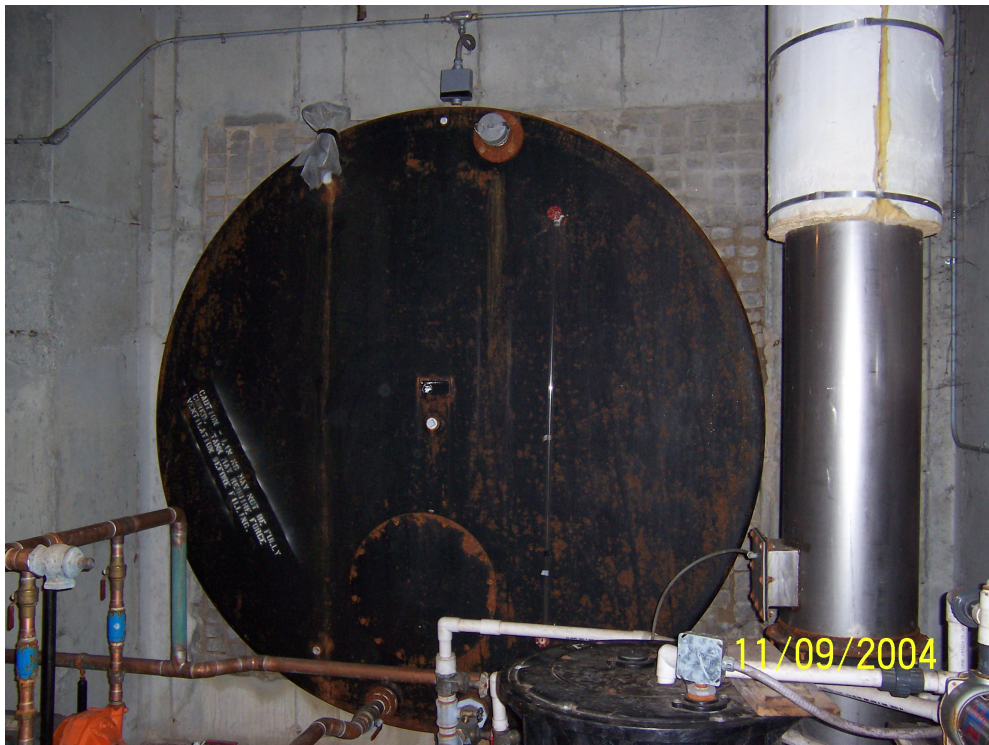
Figure 4-3. 10,000-gal Storage Tank
