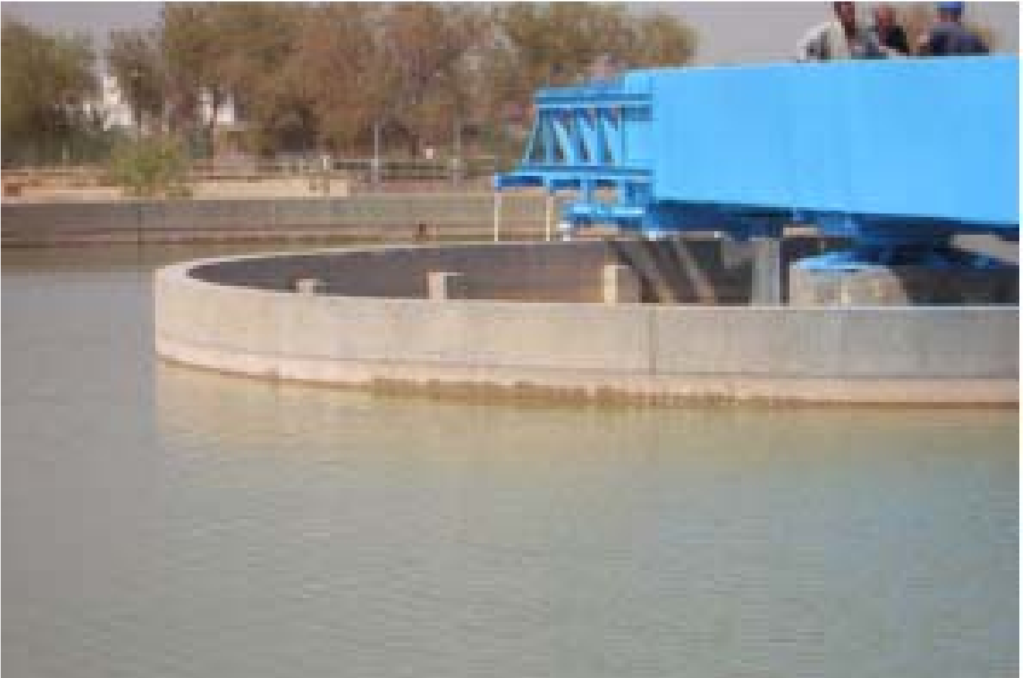
USAID is restoring and expanding a water treatment plant which will supply 170 million gallons per day to Baghdad's potable water supply.
