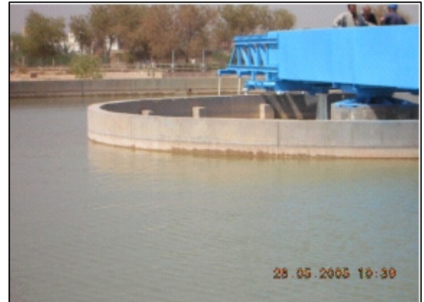
USAID is restoring and expanding a water treatment plant which will supply 170 million gallons per day to Baghdad's water supply.
