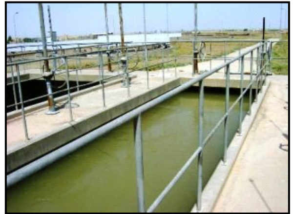
Tank for collecting water before treatment at a USAID water treatment plant rehabilitation project
