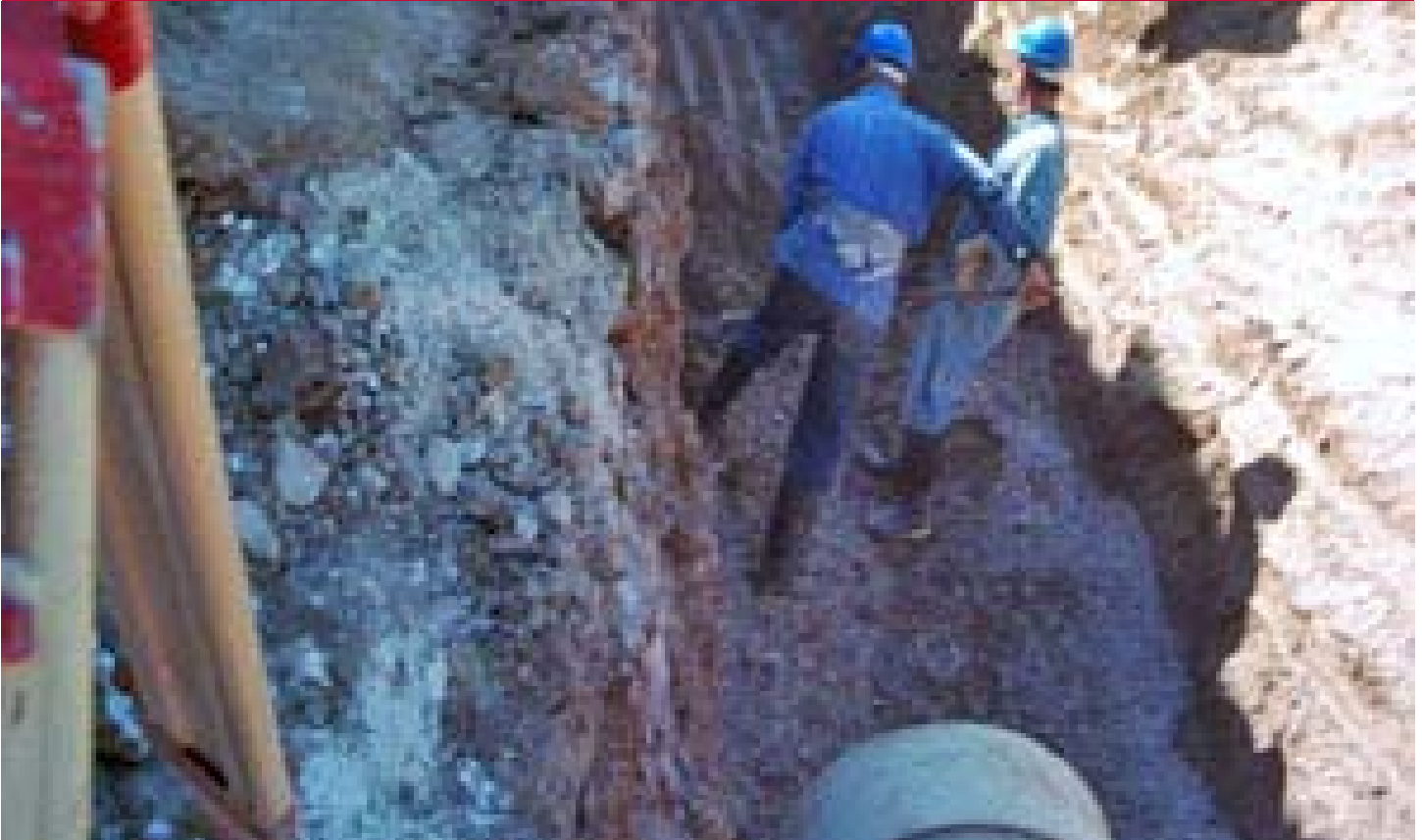
Above: Workers spread pipe bedding material as part of a project that is installing a new sewage trunk line in Baghdad.
