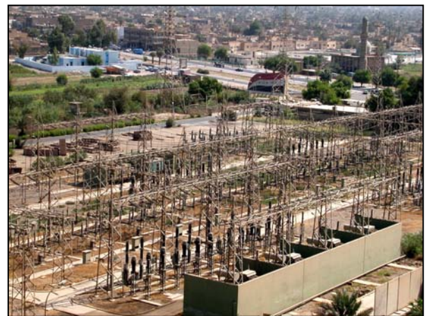
Baghdad's Doura power plant. USAID Photo.
