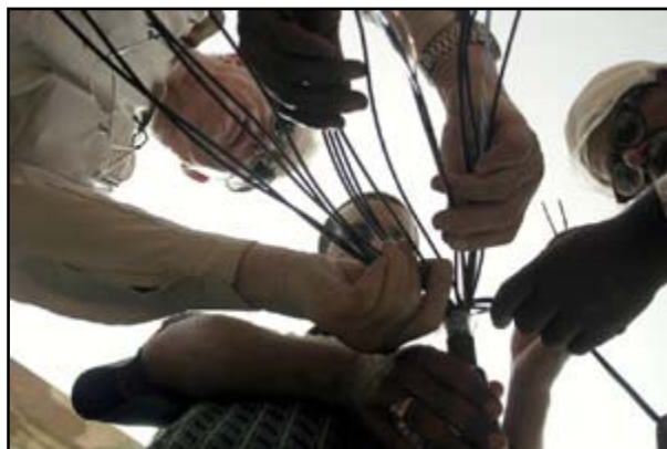
Workers inspect cables at Umm Qasr, Iraq Photo courtesy of Bechtel National, Inc.
