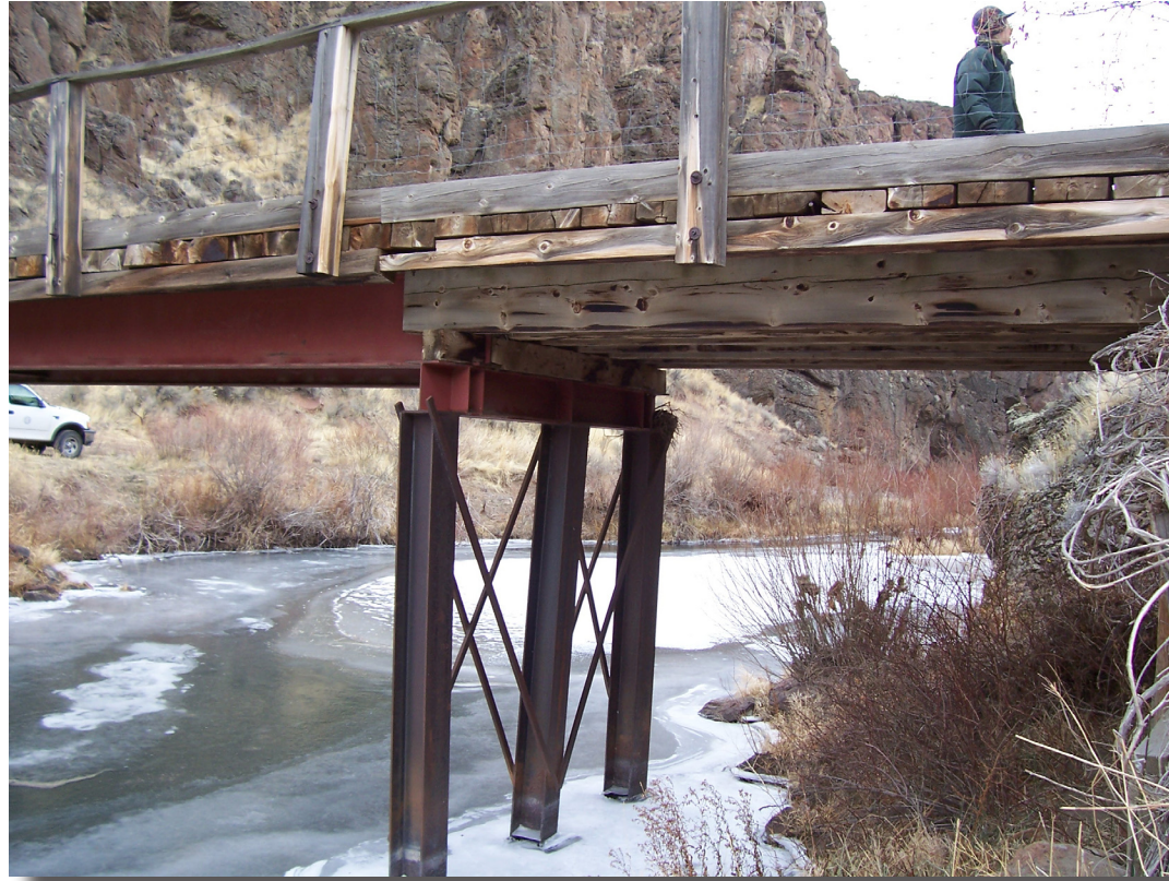
PHOTO 1 - Mid-stream pier to be removed. Photo taken from the southern bank at the SW corner of the existing bridge.
