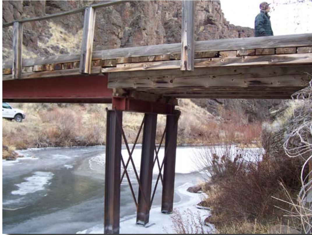
PHOTO 1 - Mid-stream pier to be removed. Photo taken from the southern bank at the SW corner of the existing bridge.
