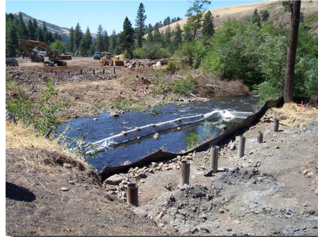
PHOTO 2 - Photo of a similar work area isolation structure on the Umatilla River.
