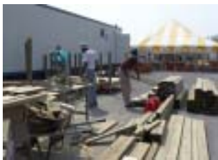
At left, workers build a temporary Post Office for Pass Christian, MS, which was completely destroyed by Hurricane Katrina.
