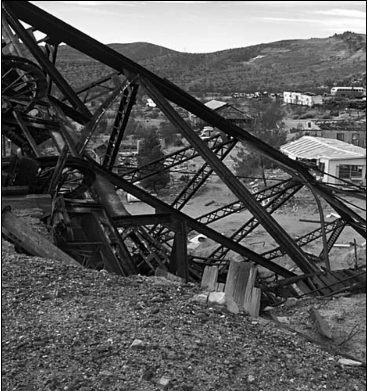
An unstable structure at the abandoned Kelly Mine in California.
