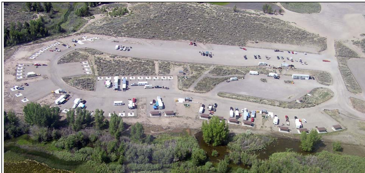
Egin Lake Recreational Site, Idaho. Phase II was completed in June 2005. BLM added several amenities to the recreation site, including power, water, site furnishings, picnic shelters, day use area, recreational vehicle dump station, and horse hitching posts.
