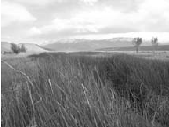
Road grade and channel restoration work at Fish Slough in Bishop, California, is dramatically improving habitat for many species, including the endangered Fish Slough milk vetch.
