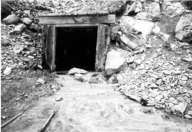
An abandoned mine adit leaking contaminated water. This adit, located in Colorado, has since been plugged using AML funds.
