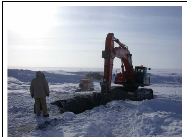
BLM's 2007 request includes funds to continue the remediation of old government-owned facilities on the North Slope of Alaska. In this picture, BLM contractors are removing the contents of a pit at the Dalton well in 2005. The contents of the pit represented a potential threat to the marine environment near the pit.
