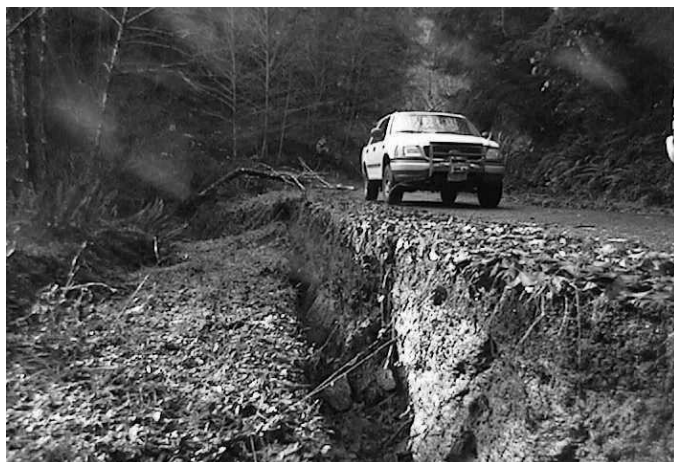
Repair of failed culverts, such as this one on a BLM road in Western Oregon, is an important function of the annual maintenance program.
