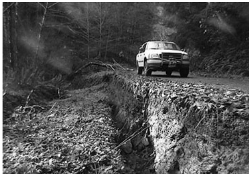
Lack of adequate annual maintenance caused a culvert to become plugged resulting in the failure of the roadside fill.
