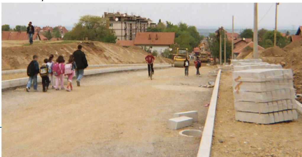
This road in Serbia is being repaved with funding supported by a USAID credit guarantee
