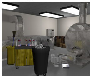
Figure 4: Improper Storage in Air Handling Room
