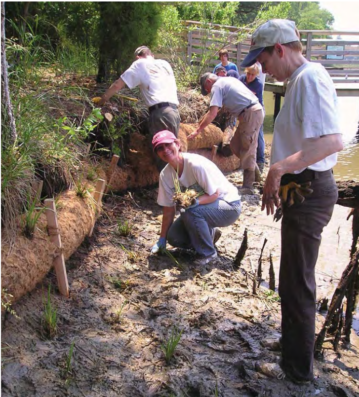
Volunteers install coconut fiber logs along a shore at Hoffler Creek Wildlife Foundation to reduce erosion. The logs were planted with wetland grasses for added habitat value as well as providing added erosion protection.
