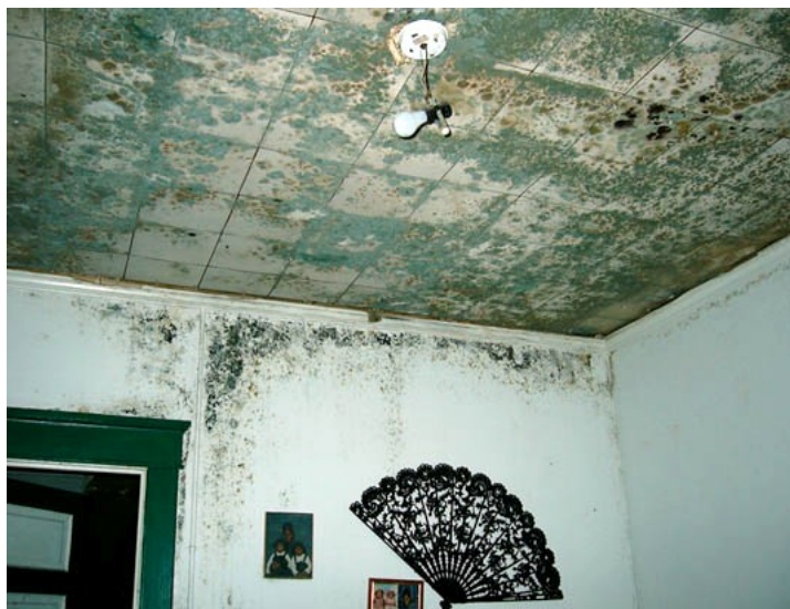
Mold growing on the ceiling and walls of a house after Hurricane Katrina
