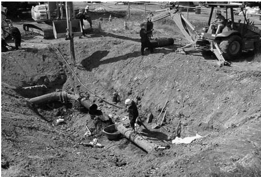
Workers help to clean up spill near Whatcom Creek.
