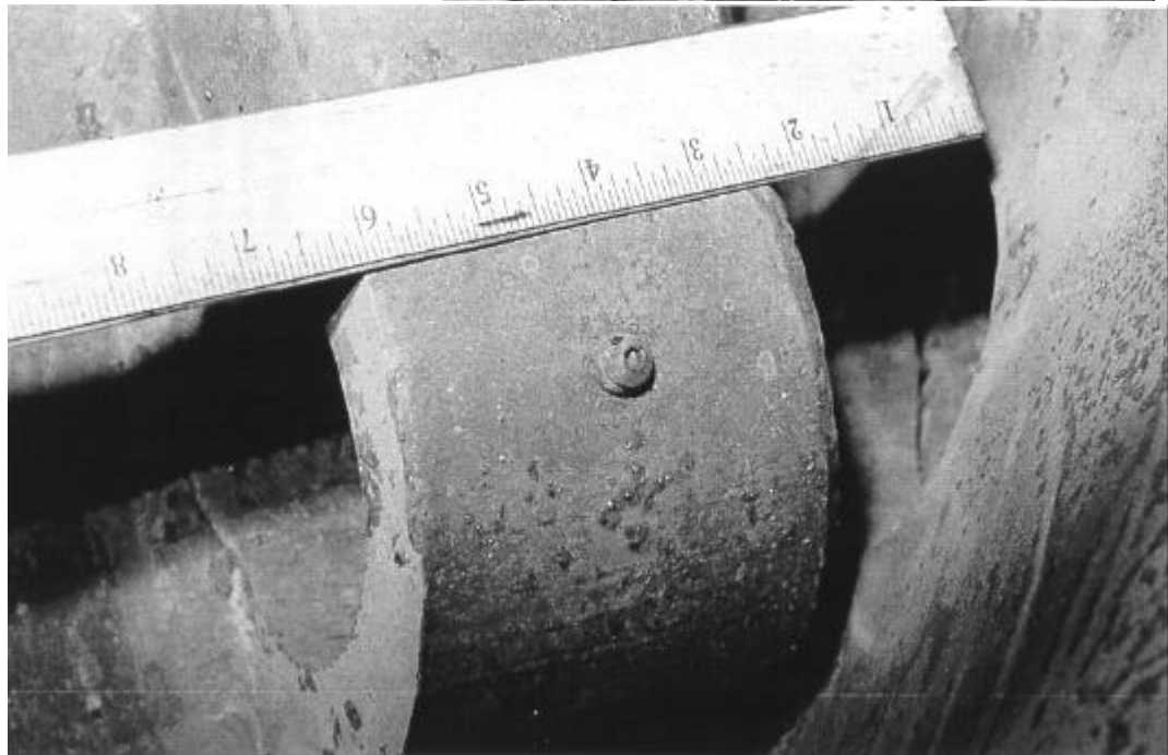
Figure E-12: Photograph shows the head of the machine screw protruding from the portion of the fractured pin. The pin is shown extended slightly out from the surface of the flange, or disk “ear”, from which the valve shaft was ejected.
