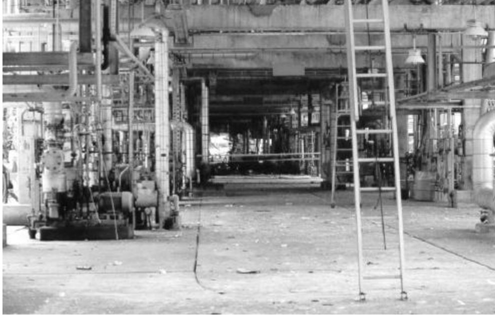
Figure E-5: Photograph looking down pipe alley (passable area underneath pipe rack) where explosion occurred.
