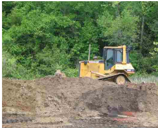
D6 dozer constructing the settling basin that will capture contaminated sediments before they get into Sutton Branch and Big Creek.
