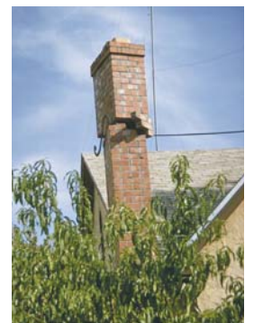
This chimney broke and nearly fell in the 1969 magnitude 5.6 Santa Rosa earthquake (photo courtesy NISEE).
