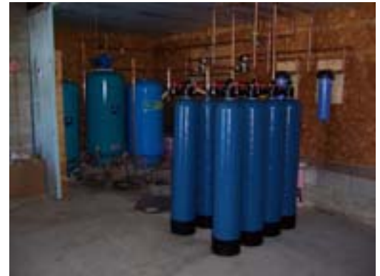
Springbrook MHPs' new arsenic water treatment equipment
