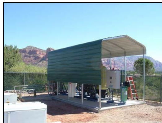
Valley Vista's new arsenic water treatment equipment
