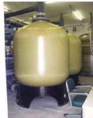
Vale's new arsenic water treatment equipment
