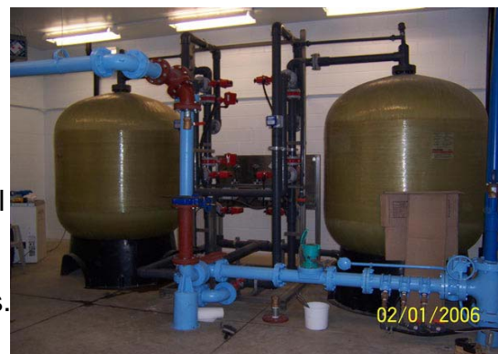
Stewart's new arsenic water treatment equipment
