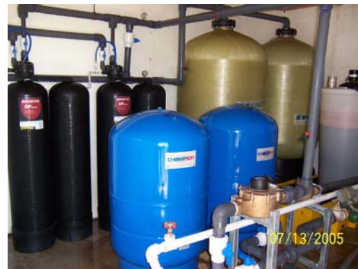
Trailer Park's new arsenic water treatment equipment
