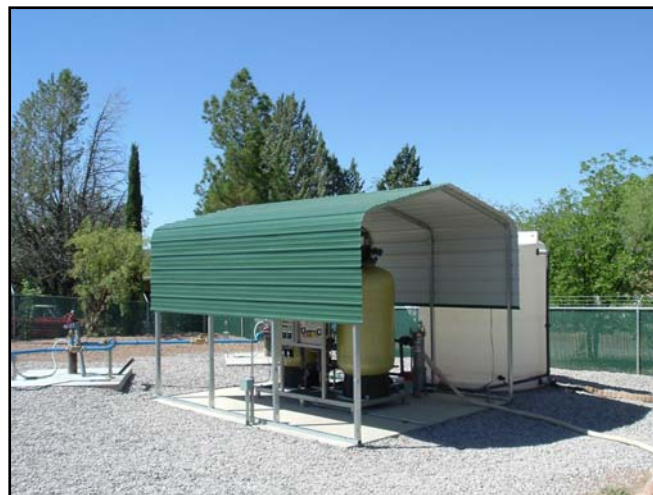
Rimrock's new arsenic water treatment equipment
