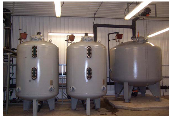
Pentwater's new arsenic water treatment equipment
