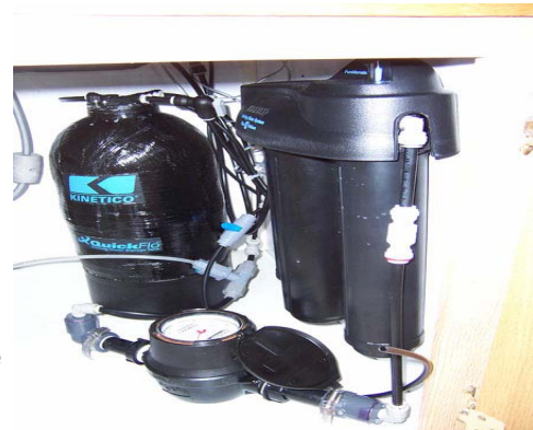
Sunset Ranch's new arsenic water treatment equipment
