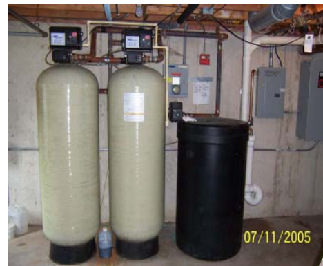
Village on the Pond's new arsenic water treatment equipment
