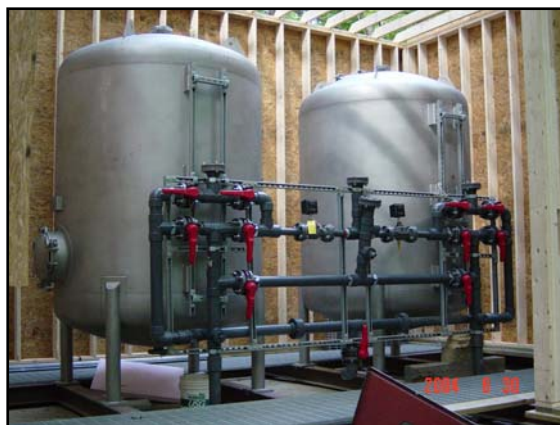
Bow's new arsenic water treatment equipment
