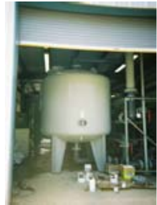
United Water System's new arsenic water treatment equipment
