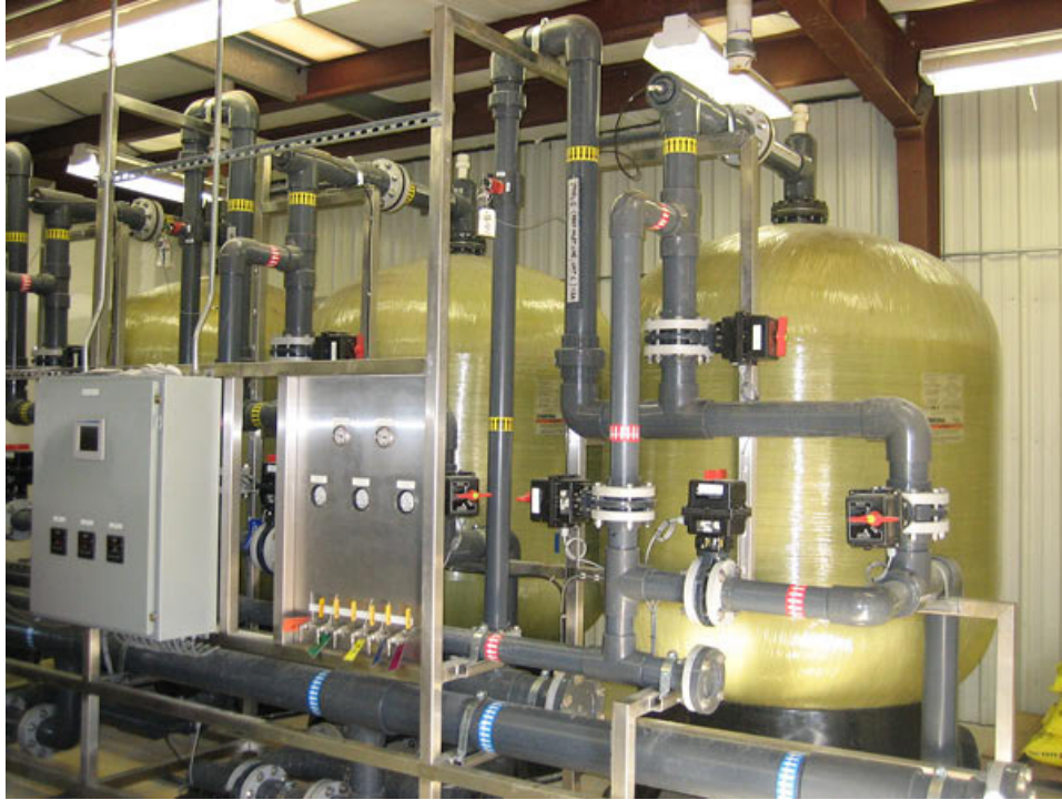
Figure 4-8. Photograph of APU-450 Arsenic Removal System
