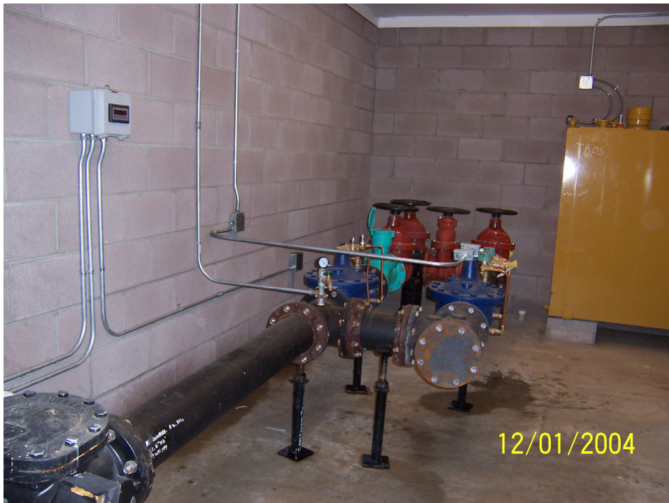
Figure 4-2. Inside of Well 8 Pump House
