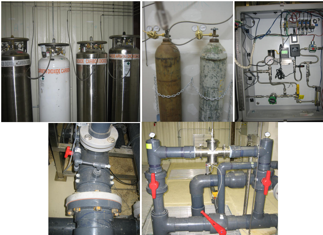
Figure 4-12. Carbon Dioxide Gas Flow Control System for pH Adjustment (Clockwise from Top Left: CO 2 Supply Assembly with Four 380-lb Dewars and Two 50-lb Cylinders; pH Control Panel; Sanitary Cross and CO 2 Loop; and Port for pH Probe)
