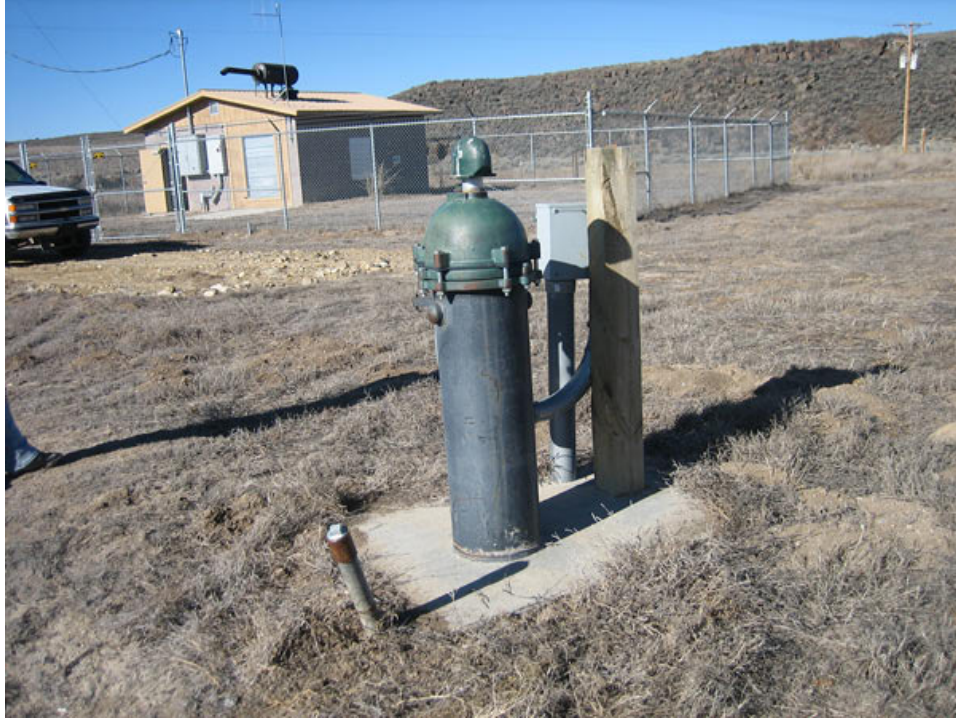
Figure 4-1. Well 8 Wellhead with Pump House in Background
