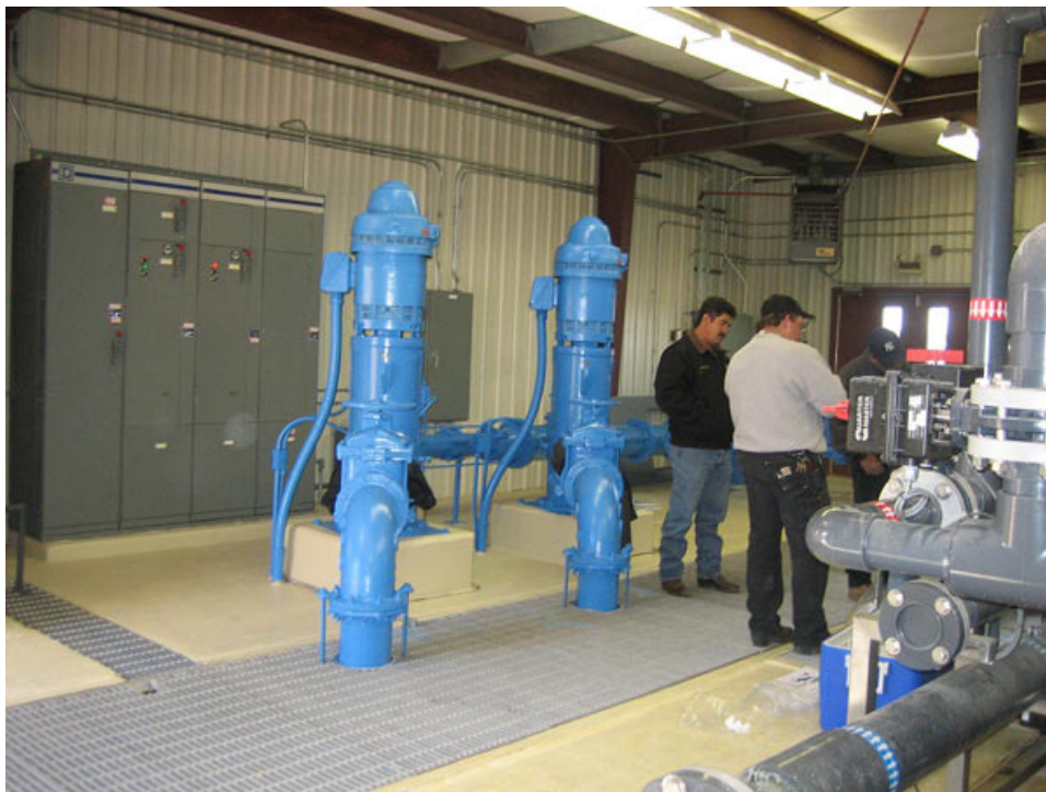
Figure 4-14. Modified Booster Pump Station
