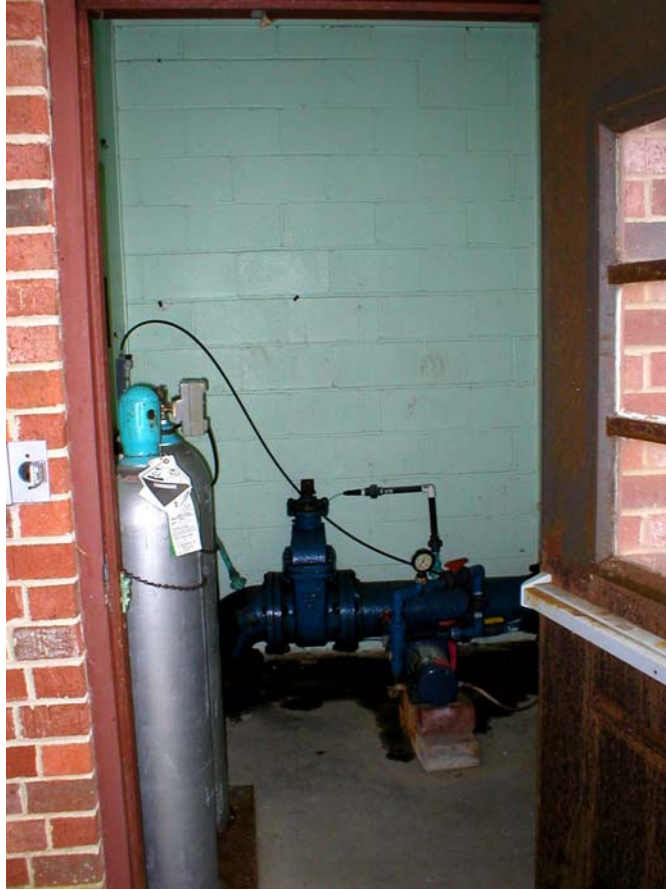
Figure 4-2. Chlorine Gas System at Well No. 1
