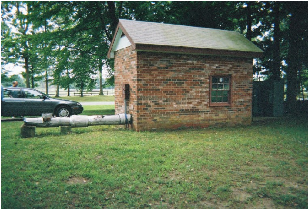
Figure 4-1. Existing Well House No. 1
