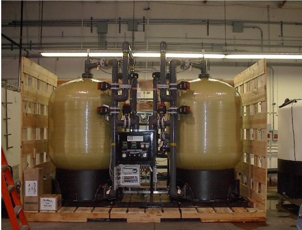
Figure 4-3. APU-300 Treatment System Prior to Shipment
