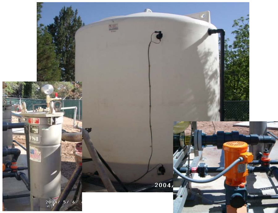
Figure 4-4. Backwash Recycling System Components (From Left: Backwash Bag Filter; 3,000-gal Storage Tank with Level Sensors; and Recycle Pump)
