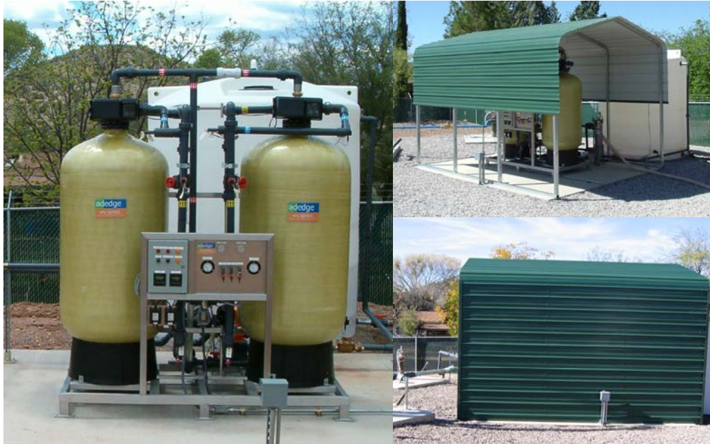
Figure 4-6. System Enclosure (Clockwise from Left: System Installed on Concrete Pad in April 2004; Sun Shed Built in May 2004; and Enclosure Completed in December 2004)
