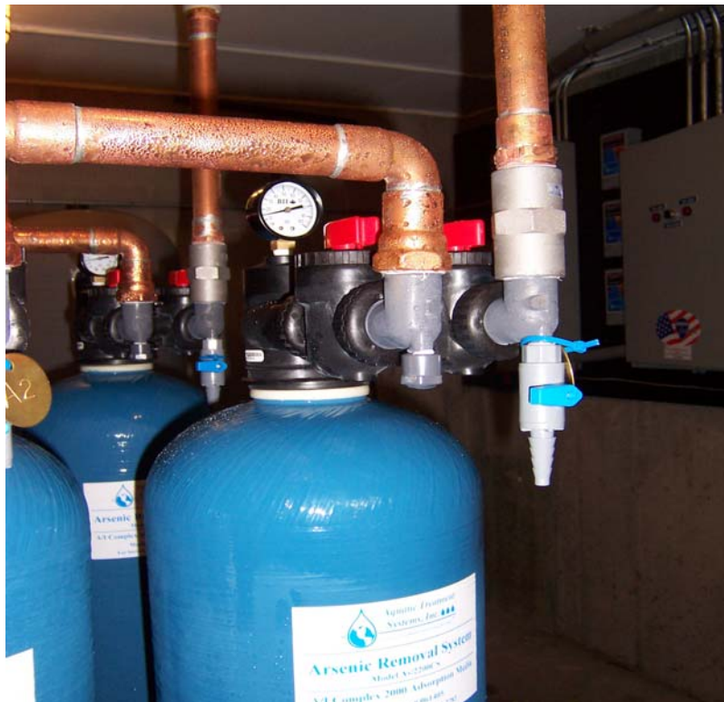
Figure 4-6. Close-up View of a Sample Tap (TE), a Pressure Gauge, and Copper Piping at End of Treatment Train A
