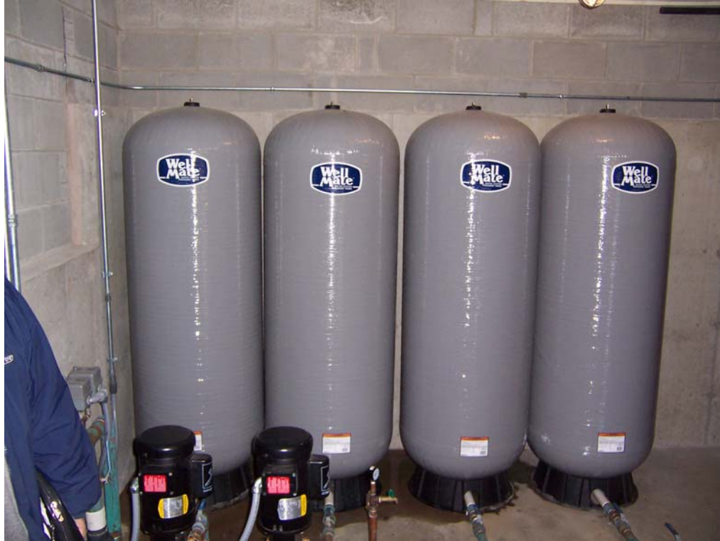
Figure 4-2. Pre-Existing Pressure Tanks and Booster Pumps
