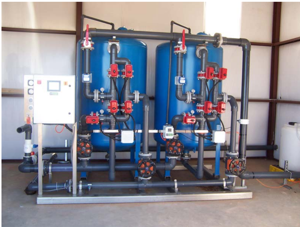
Figure 4-6. Adsorption System Valve Tree and Piping Configuration
