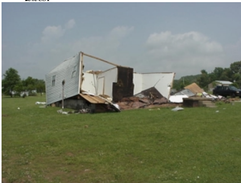
Damage in Atwood from a F1 tornado which struck on May 4th.
