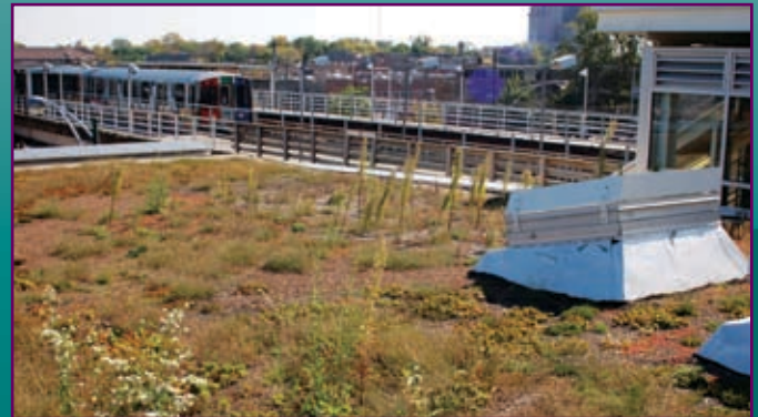
Bethel Center's green roof reduces stormwater runoff, and photovoltaic cells provide clean energy. The center also provides direct access to the Green Line "EI" stop through a connecting bridge.
