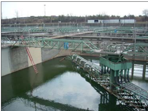
Final clarifiers and influent baffles that increase the capacity of the Passaic Valley Sewerage Commissioners plant in Newark, New Jersey (EPA OIG photo).
