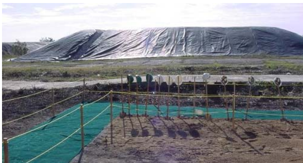
The contaminated soil mound contained within a high density polyethylene cap at the Escambia Treating Company Superfund site (EPA OIG photo).
