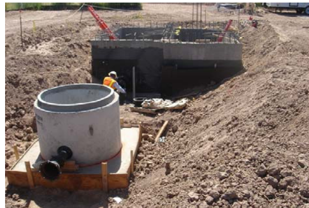
Construction of a wastewater treatment plant in Tornillo, Texas, funded through the Colonias Wastewater Treatment Assistance Program (EPA photo).
