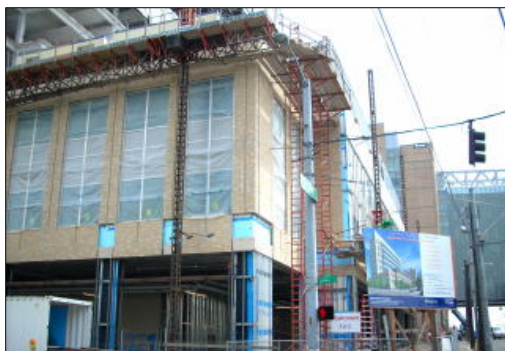
Construction taking place at a Seattle public hospital that is a cleaned-up brownfields site (EPA OIG photo).
