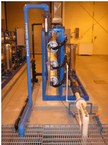
Nano-filtration system at a tribal drinking water facility (EPA OIG photo).
