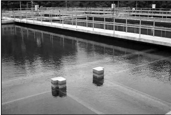
Multiple stages of treatment—including sedimentation, which is shown here—are used for sources such as surface waters, whose quality is variable.
