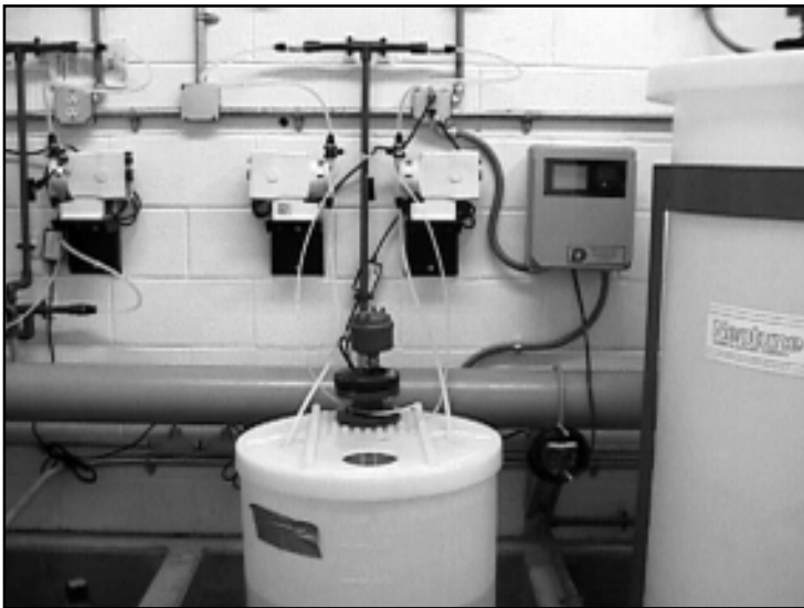
Simple chlorination treatment for a small ground water system.
