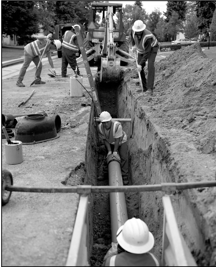
Repair or replacement of distribution system components can create a potential source of contamination.
