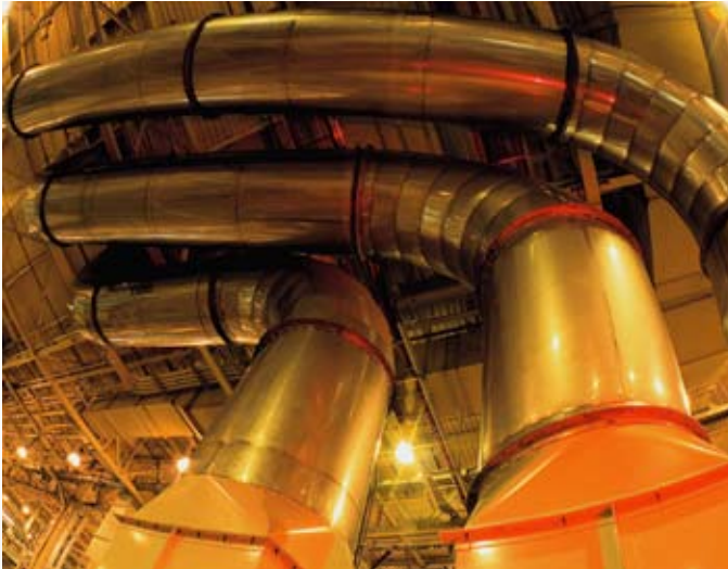
Ceiling ducts draw wasted heat from the furnaces, transporting it to cooler areas of the DMMI facility
