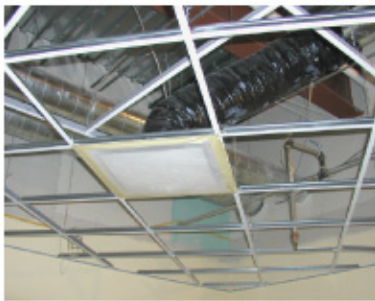
During construction, the HVAC system and duct work were sealed on a daily basis to prevent infiltration of any dust, chemicals, or odors due to construction. Before occupancy, the system was flushed and fresh air filters were added.
