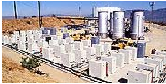
Large Scale Microturbine Application
