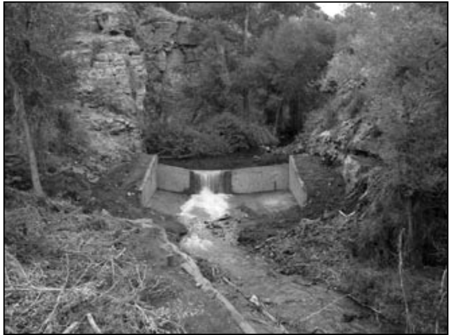
The Crooked Creek fish barrier will keep nonnative trout from migrating upstream into the native Yellowstone cutthroat trout habitat.
