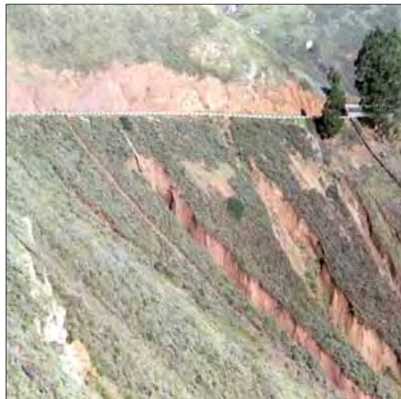
Photo 1.14 Erosion scars below Conzelman Road.
