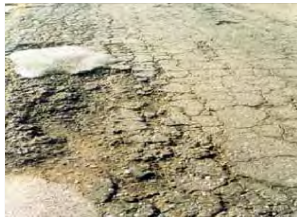
Photo 1.1. Deteriorated roadway asphalt pavement in Fort Barry.
