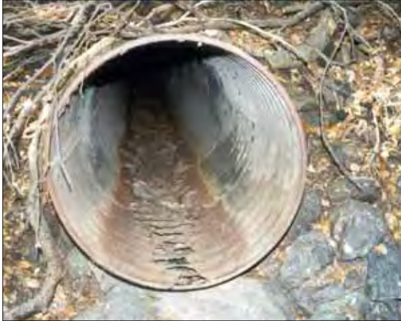
Photo 1.2. Rusted culvert under East Road.
